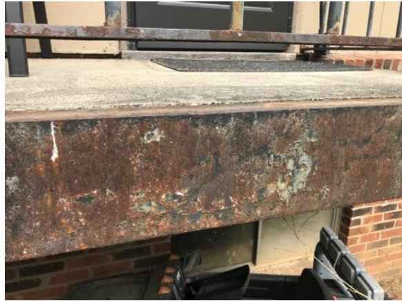
Photo 30 - Typical back porch metal floor frame - POSITIVE
